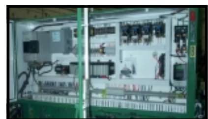
New CF Electrical Panel
